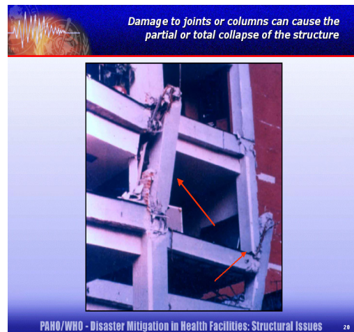
Figure 6-2: Damage to joints or columns involves structural damage that can lead to a building collapsing
